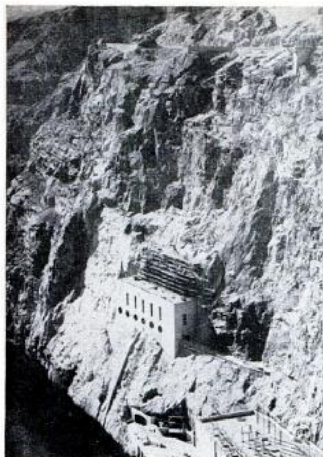
Huge rock slab hangs just above the valve house. Scaffold for the workmen was built around the slab
